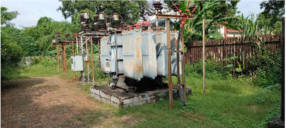
Electrical Sub Station
